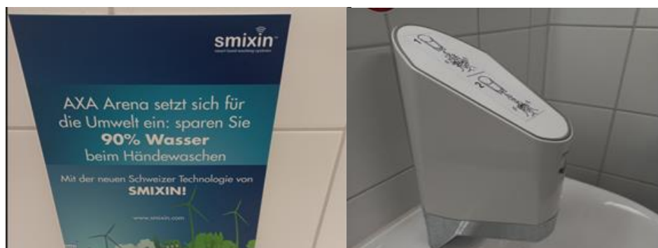
Figure 69 - Automatic dispenser of water and soap to reduce their consumption in the toilettes of the AXA Arena.
