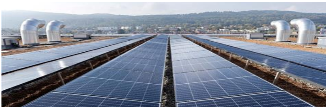
Figure 63 - Photovoltaic panels on the roof of Life Swiss Arena
